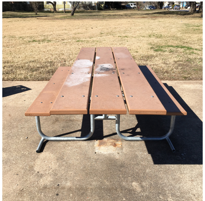
Figure 4.34 Shows the condition of picnic table
