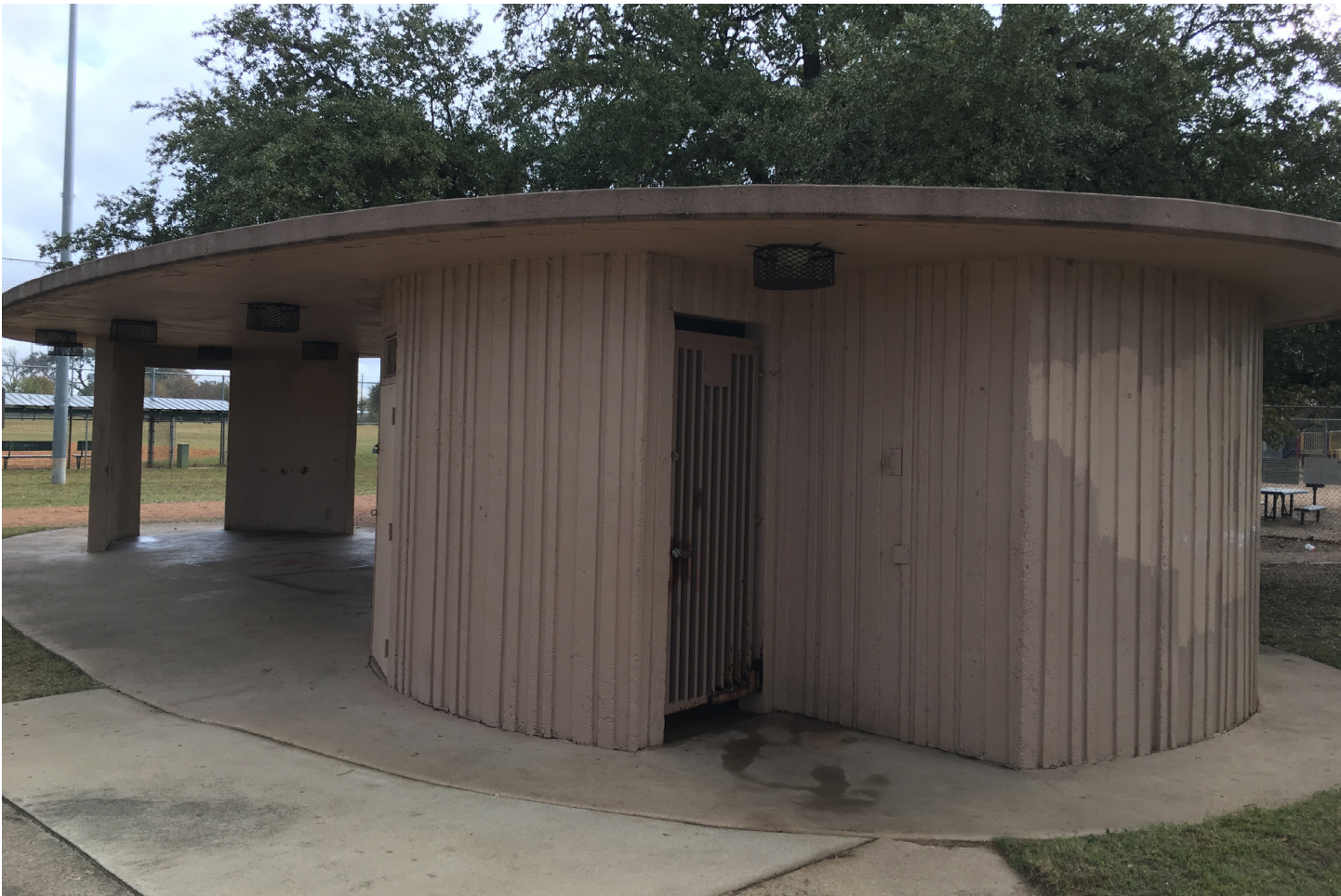
Figure 4.22 Shows the conditions of the restroom at Civitan Park
