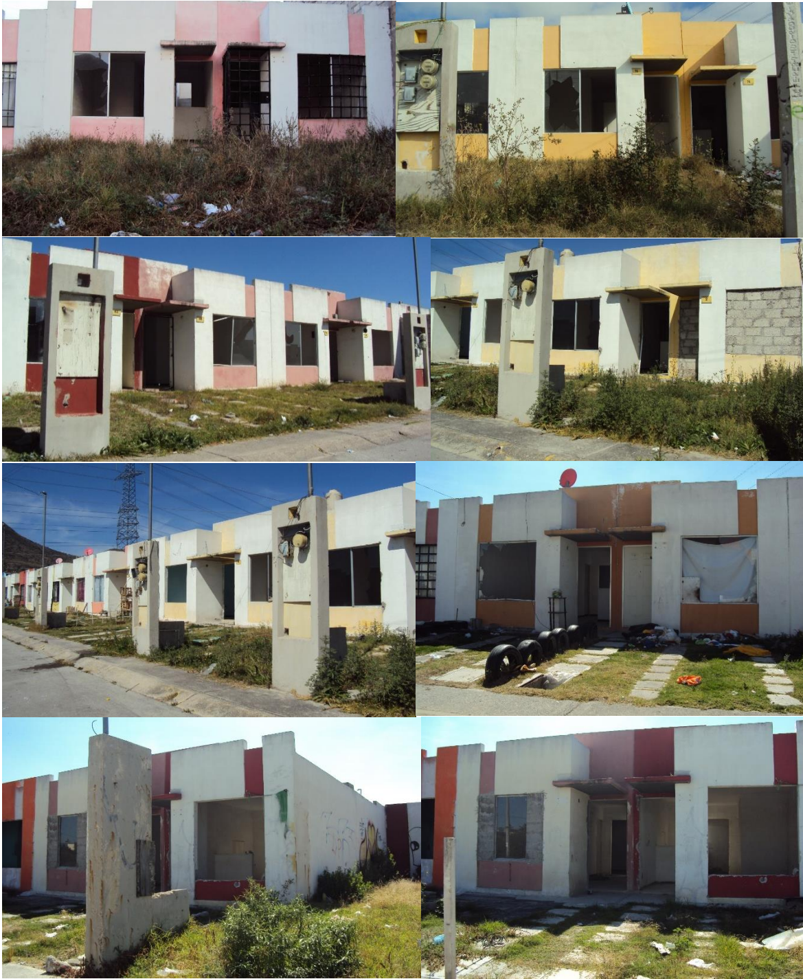
Figure 5.31: Abandoned Low-Income Housing in Santa Teresa, Huehuetoca.
