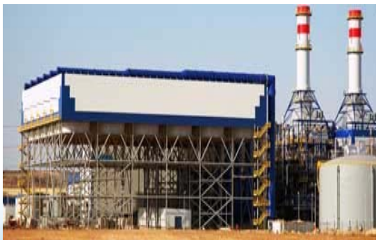
Dry-Cooled Power Plant
