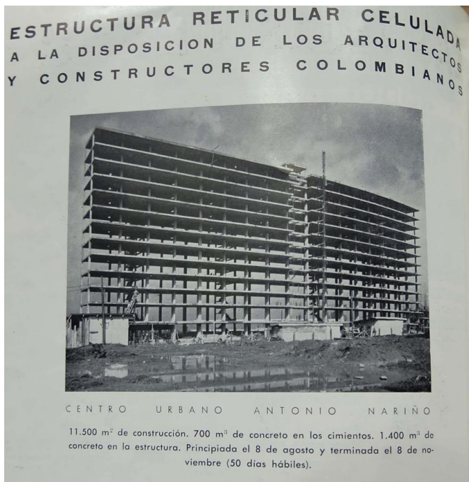
Figure 3.24. Advertisement of Cuellar, Serrano, Gómez & Cia. Ltda., of its building method "Reticular Celulado." Published in Proa 65, November 1952.
