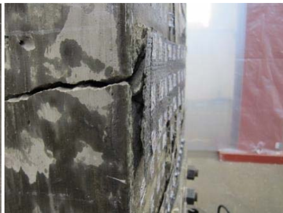
(f) Crack pattern of U5-0-0-5
