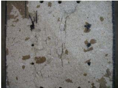
(c) Crack pattern
