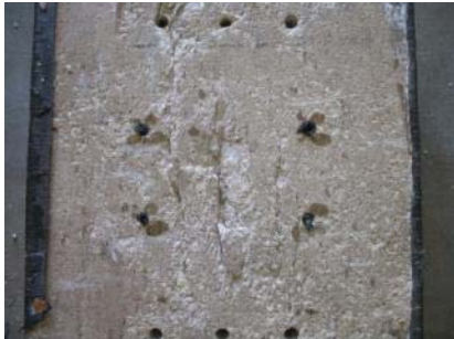
(c) Crack pattern
