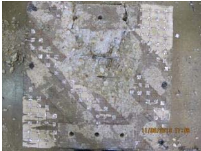
(c) Crack pattern
