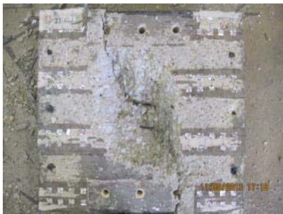
(c) Crack pattern
