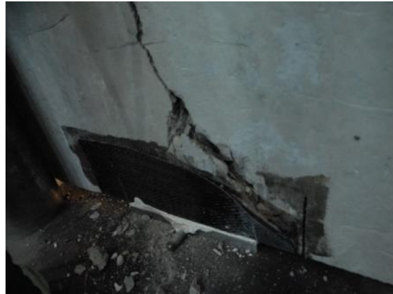
(b) Funnel-shaped concrete crushing
