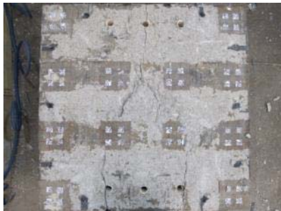
(c) Crack pattern
