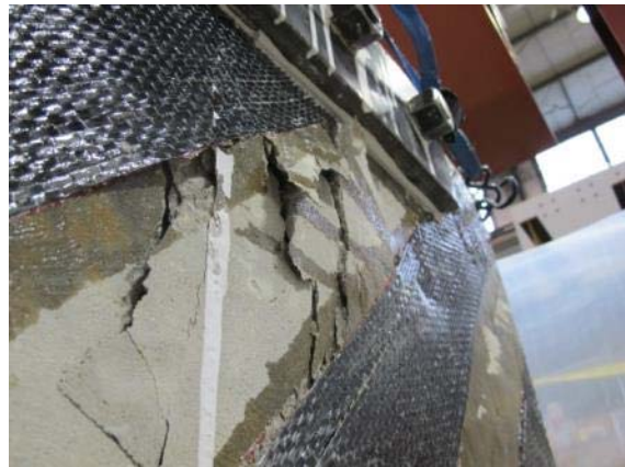
(f) Crack pattern of U5-45-0-5
