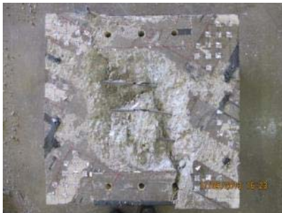
(c) Crack pattern
