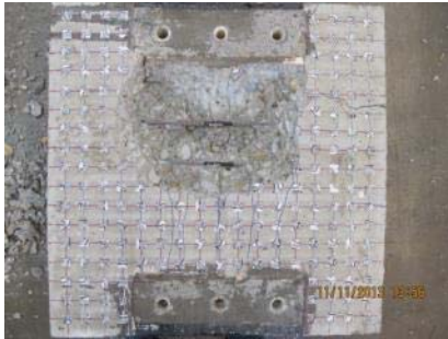
(c) Crack pattern
