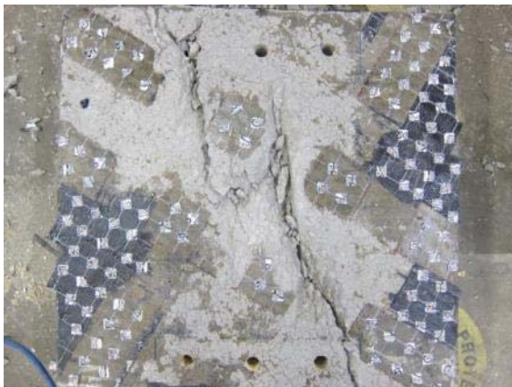
(e) Crack pattern of B5-60-0-5
