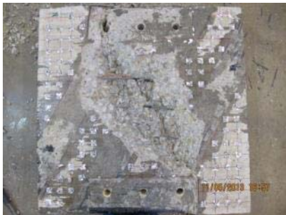
(c) Crack pattern
