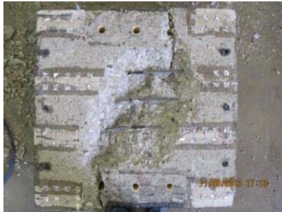
(c) Crack pattern
