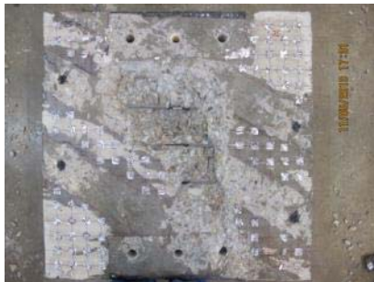
(c) Crack pattern
