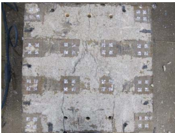
(e) Crack pattern of B5-0-0-5
