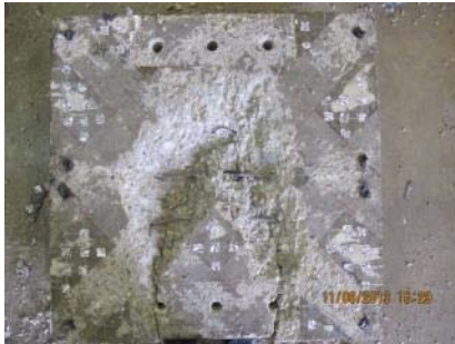
(c) Crack pattern
