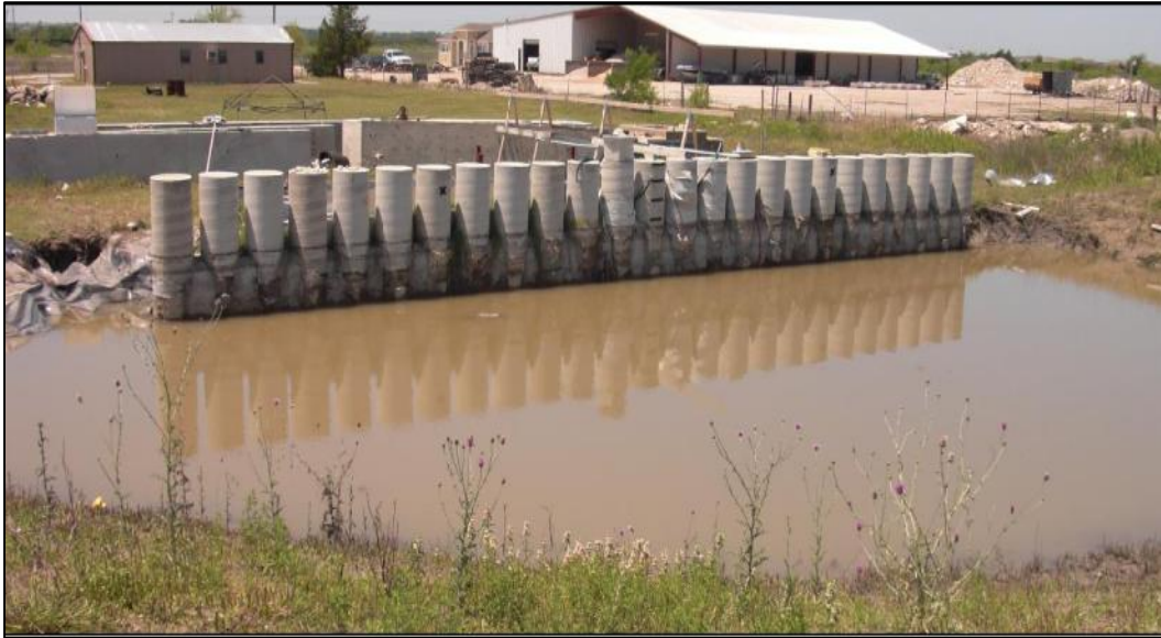
Figure 9.31: Reese wall site conditions after severe rainfall, May 6 2013 (Brown 2013)
