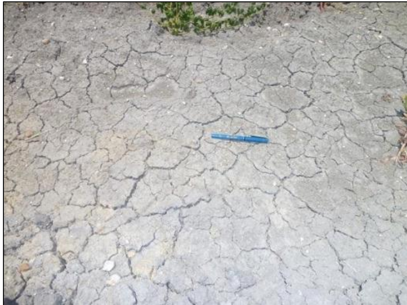
Figure 3.7: Desiccation cracks of the soil during site investigation
