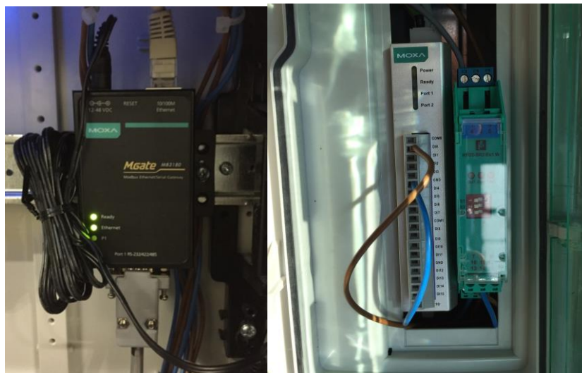
FIGURE 38. DEVICES USED TO CONNECT METERS TO THE NETWORK (MODBUS LEFT, PULSE RIGHT)
