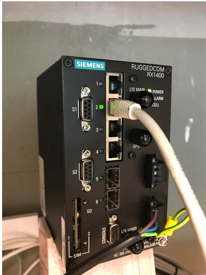
FIGURE 32. LEM INSTALLED ON THE RUGGEDCOM RX1400 AT THE FRENCH PILOT SITE
