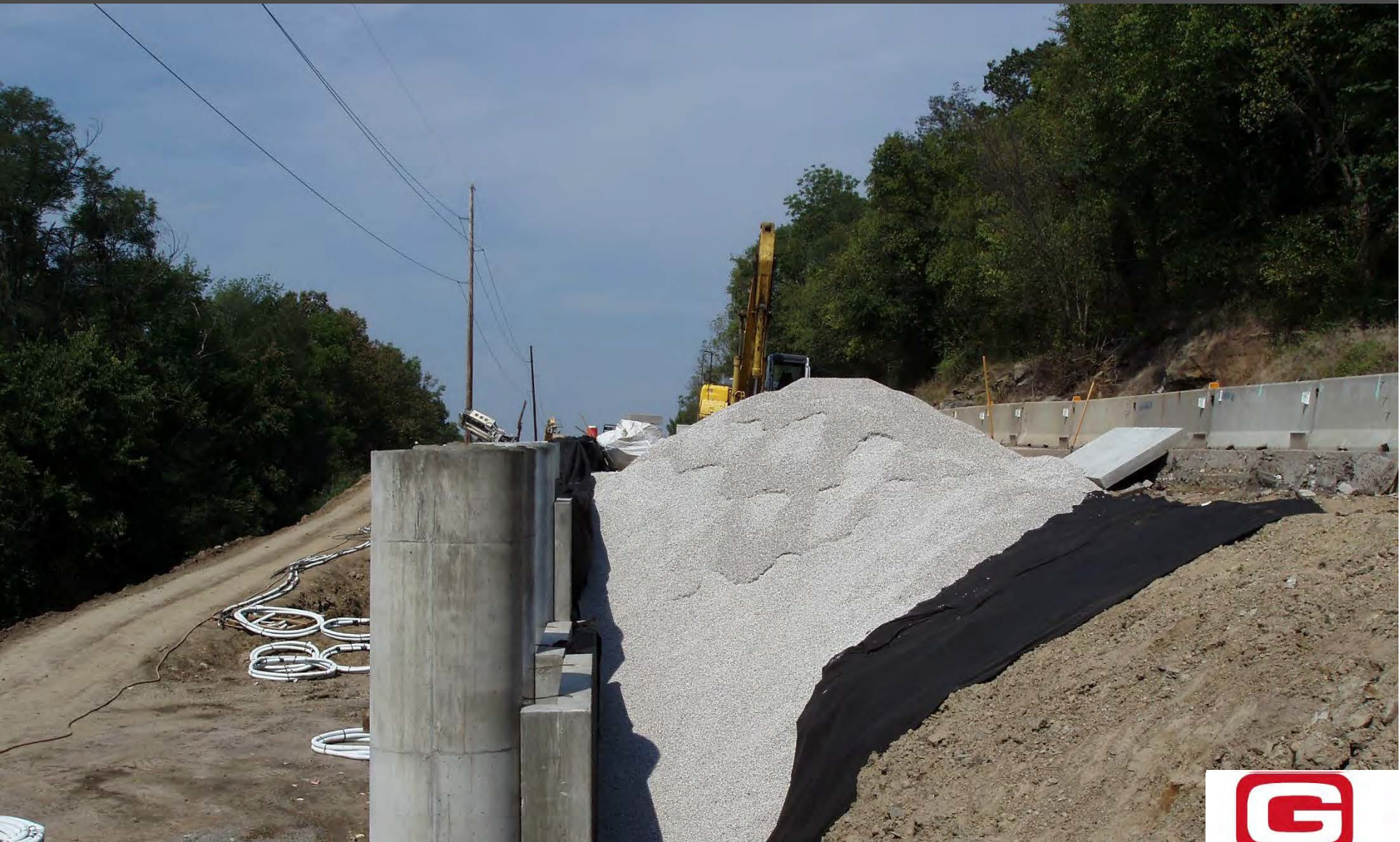
SR 66 Landslide, Perry County, Indiana
