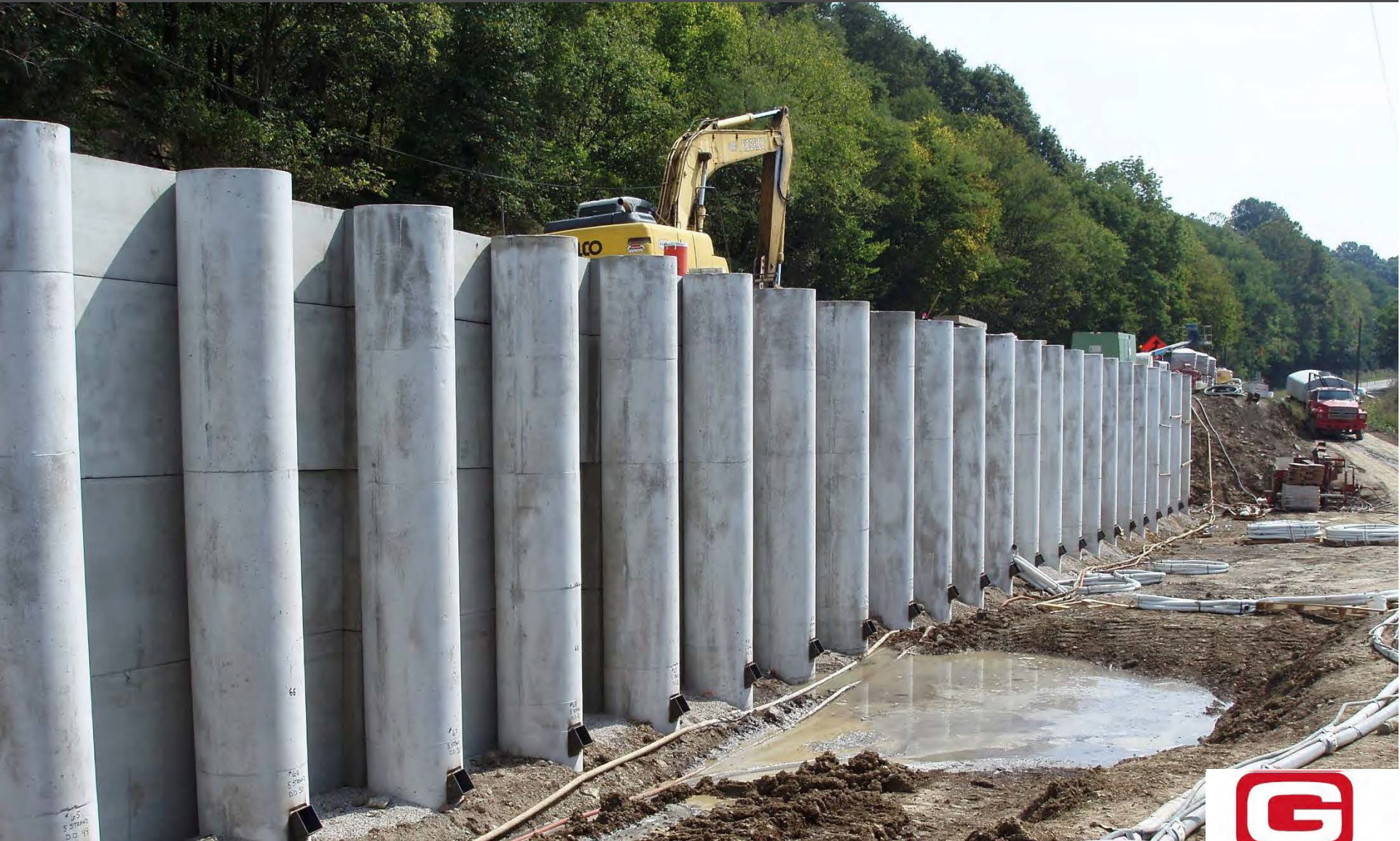
SR 66 Landslide, Perry County, Indiana
