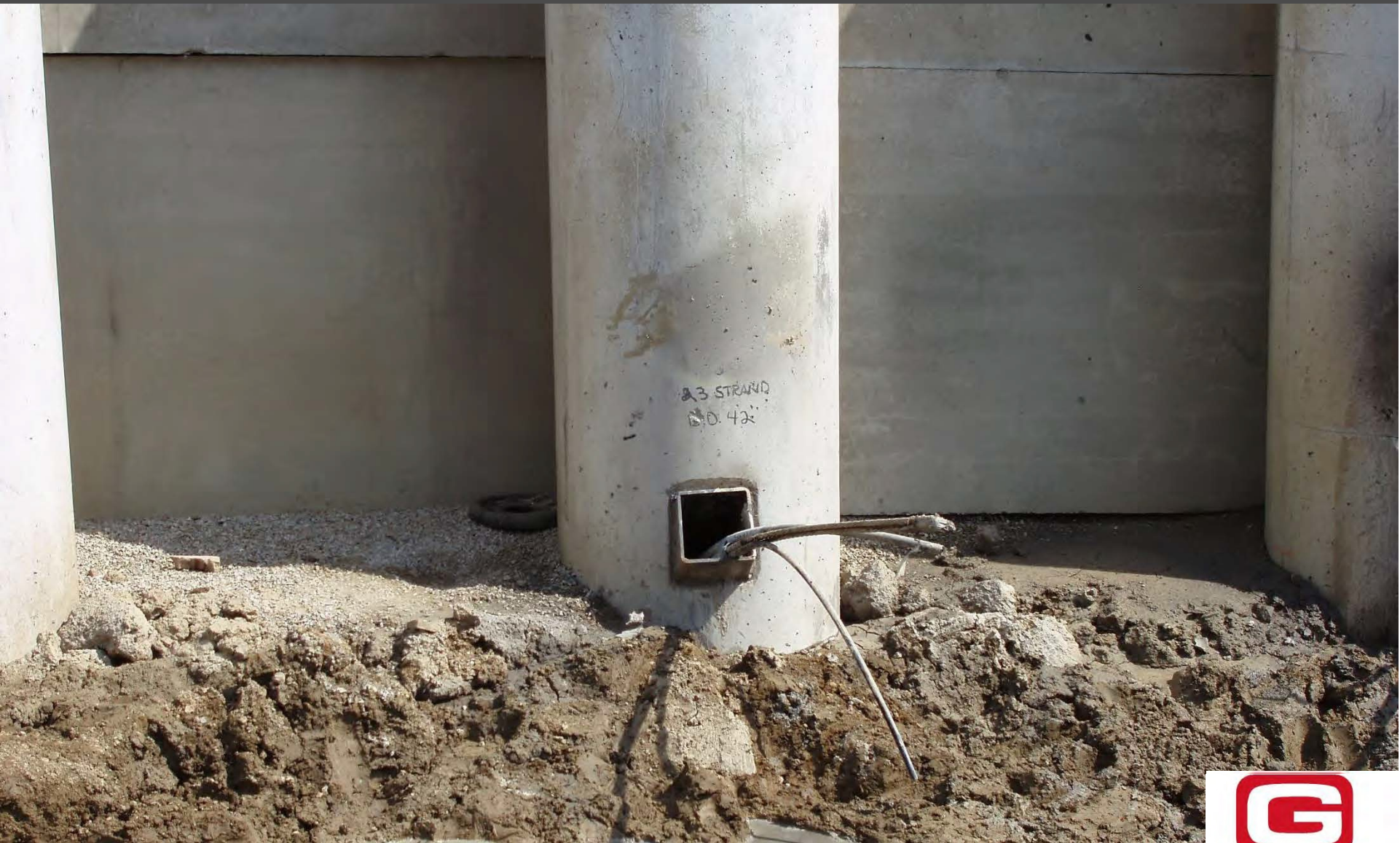
SR 66 Landslide, Perry County, Indiana
