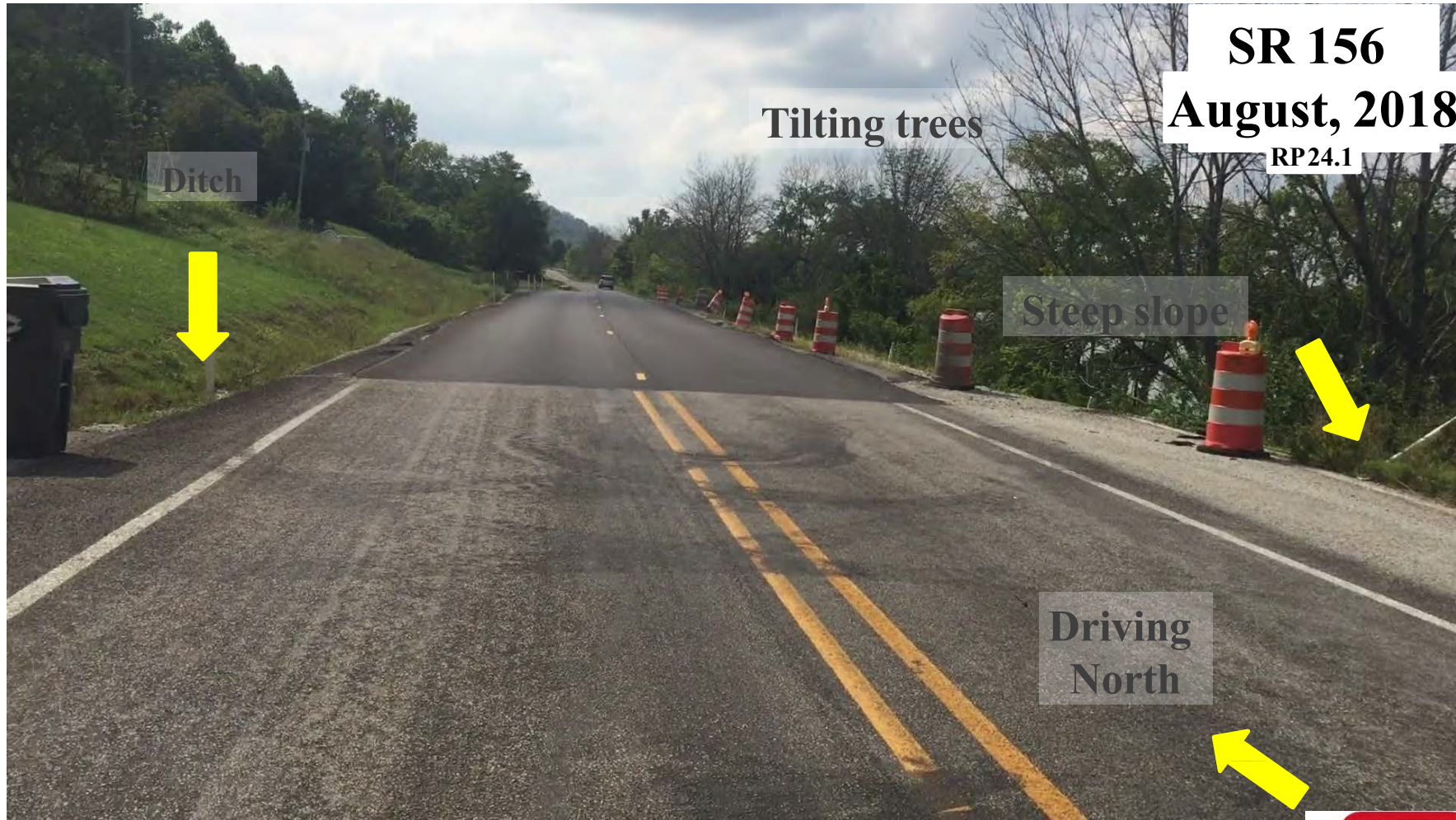
SR 156 Landslide RP 24.1
