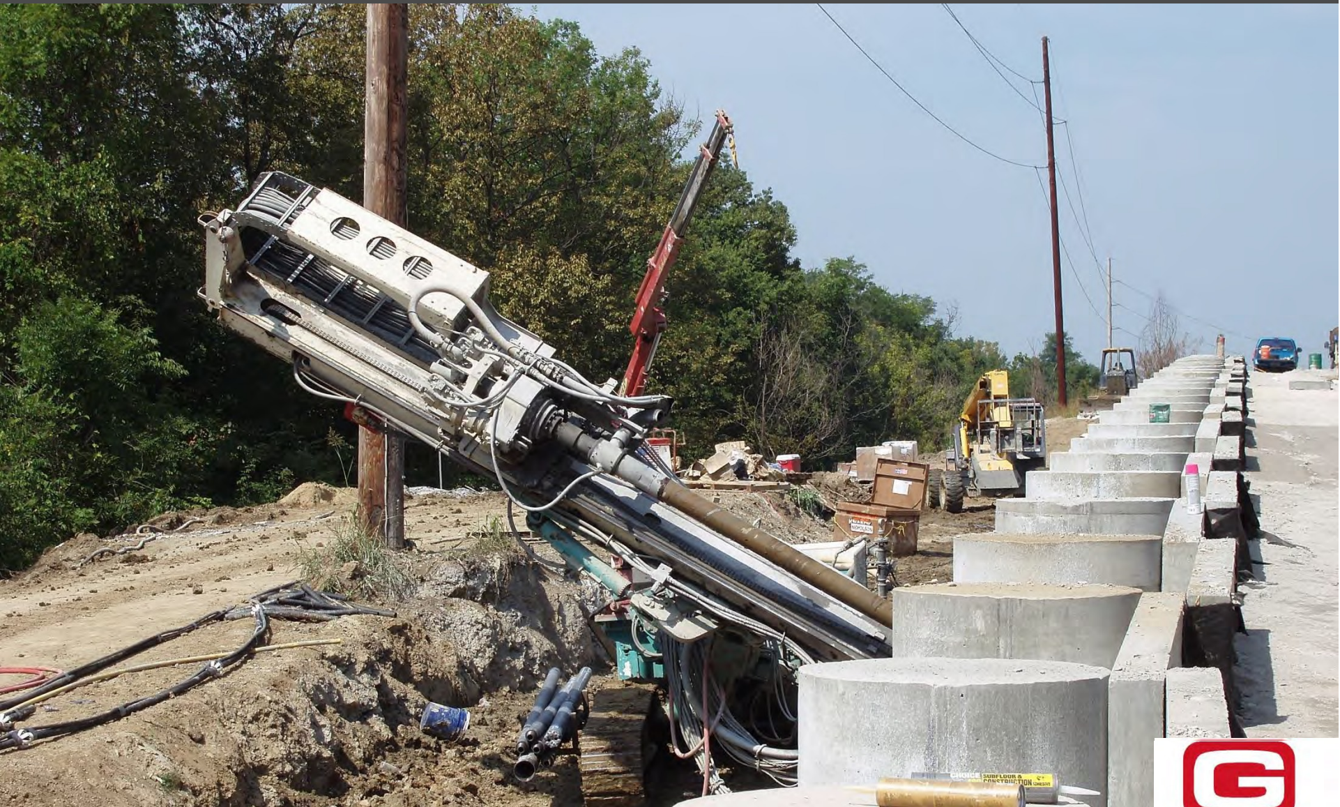
SR 66 Landslide, Perry County, Indiana
