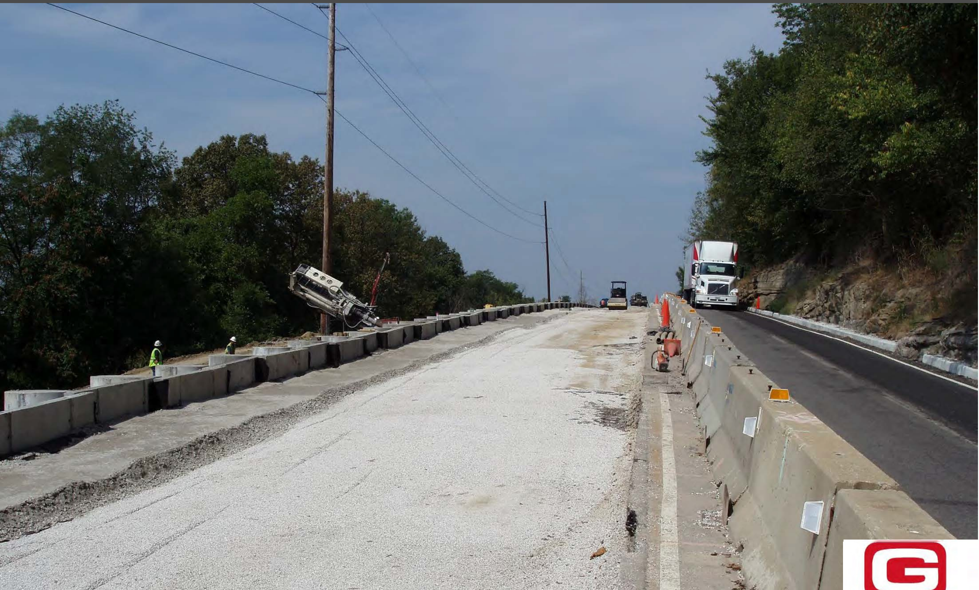
SR 66 Landslide, Perry County, Indiana
