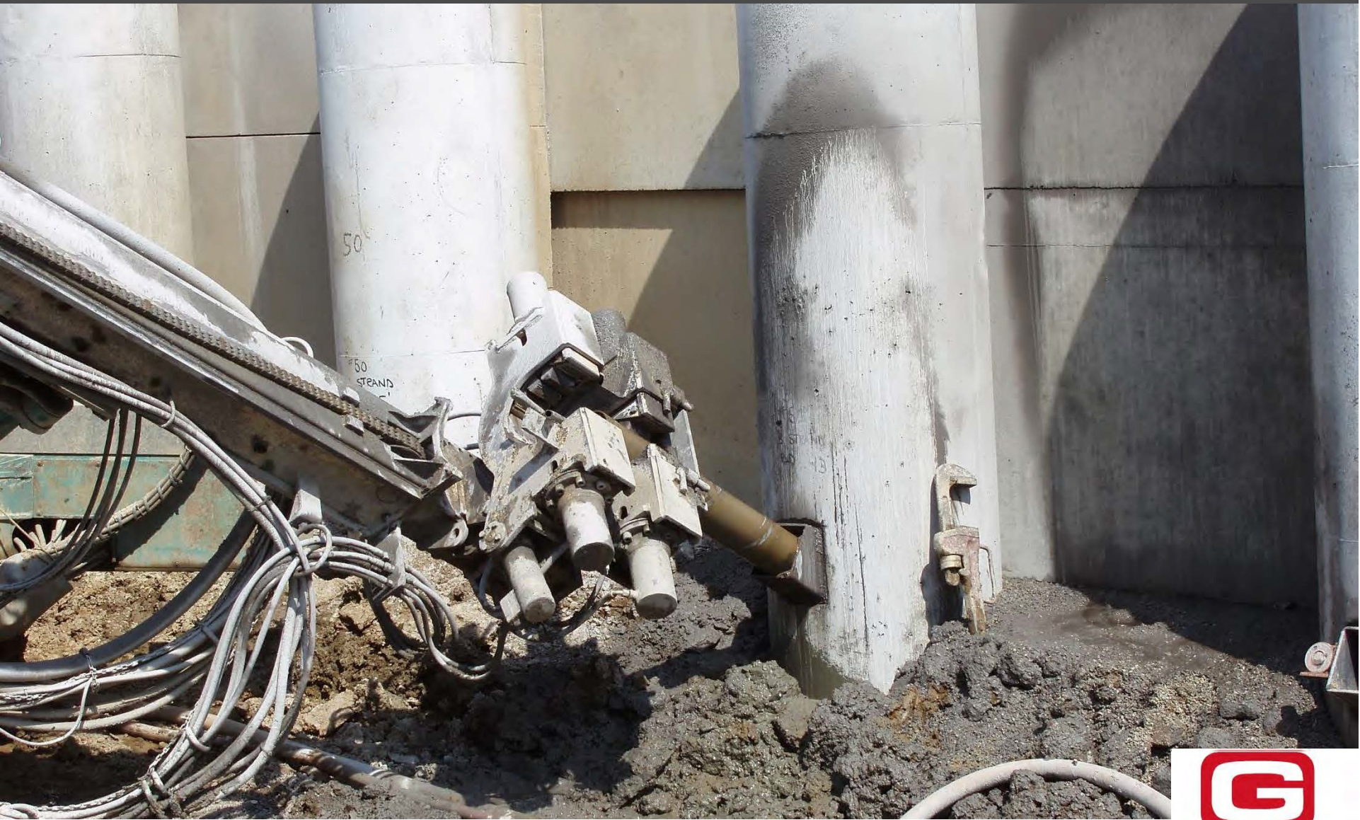
SR 66 Landslide, Perry County, Indiana
