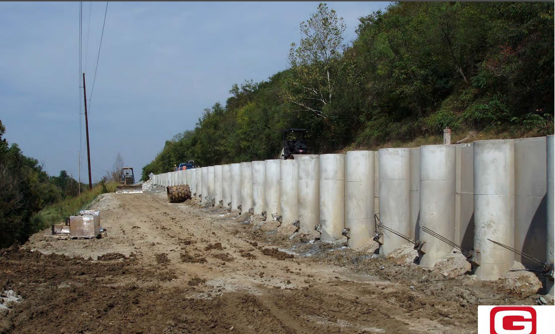
SR 66 Landslide, Perry County, Indiana
