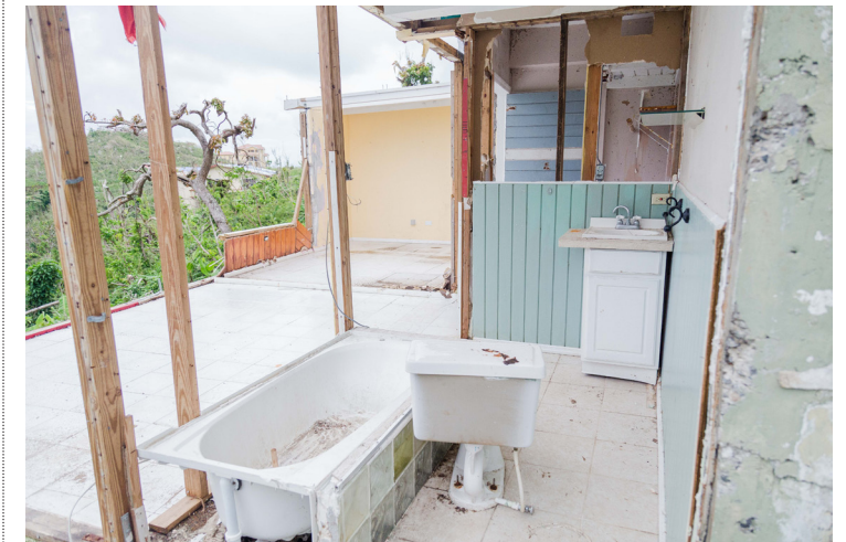
The disappeared north rooms that left the house an open sepulchre (taken months after Hurricane Irma and clean-up). Credit: Kamaal Lettsome, November 2017.
