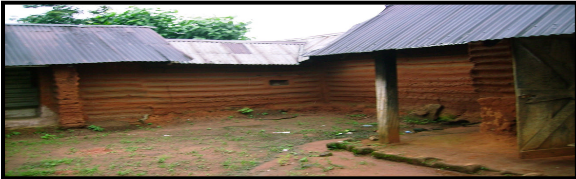
Figure 5: shows that mud walls are finished in a pattern of horizontal ribs
