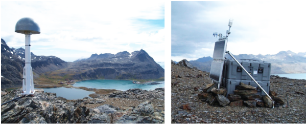
Fig. 2 GNSS antenna and radome on 1-metre mast (left) and aluminium pipe frame with electronics and auxiliary equipment (right).
