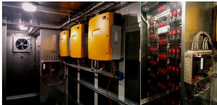
Bidirectional inverters (three-phases system)
