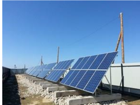
Figure 4.32 Installed 20kWp PV Plant – Yakutsk
