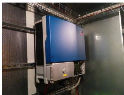
PV inverter (three-phases)
