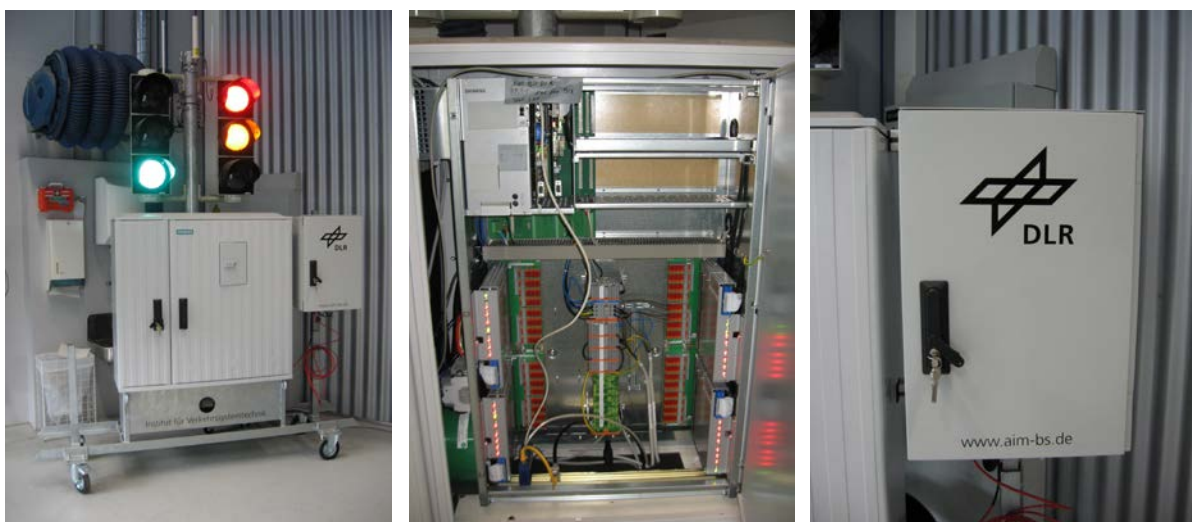
Figure 2 – Field operational test installation (left) with the signal controller Siemens C940V (middle) and the road side unit (right).
