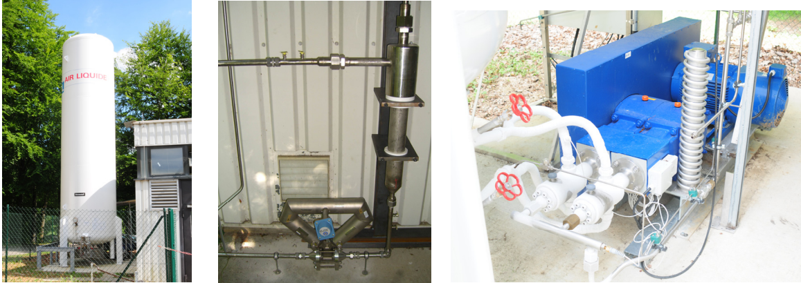
Figure 5: Liquid Nitrogen tank, mixer and cryogenic piston pump.
