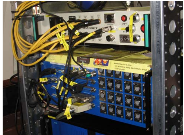
Figure 16 Auxiliary Rack: Intercomm, Breakoutbox, ALC control PC, Multi Input Recorder PC.
