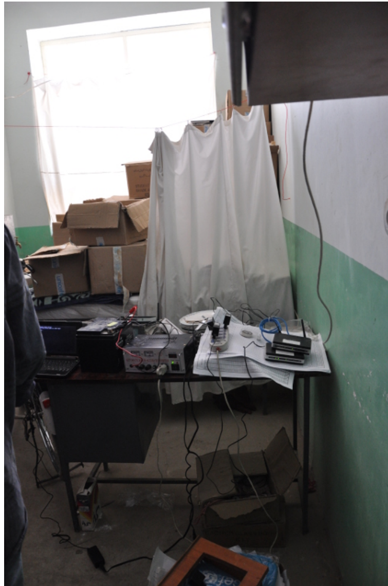
Figure 7.1: Server-room at School One with a car battery, an inverter and a multi-socket connected to them. (source: the author)
