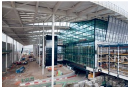
Top: The installation process, 2014. Above: A view of the forecourt area as Terminal 2A is constructed, 2012
