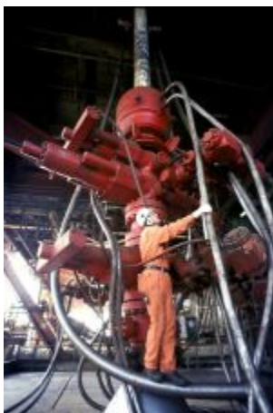
Figure 15. Hydraulic system on Statfjord B. Photo: Statoil.
