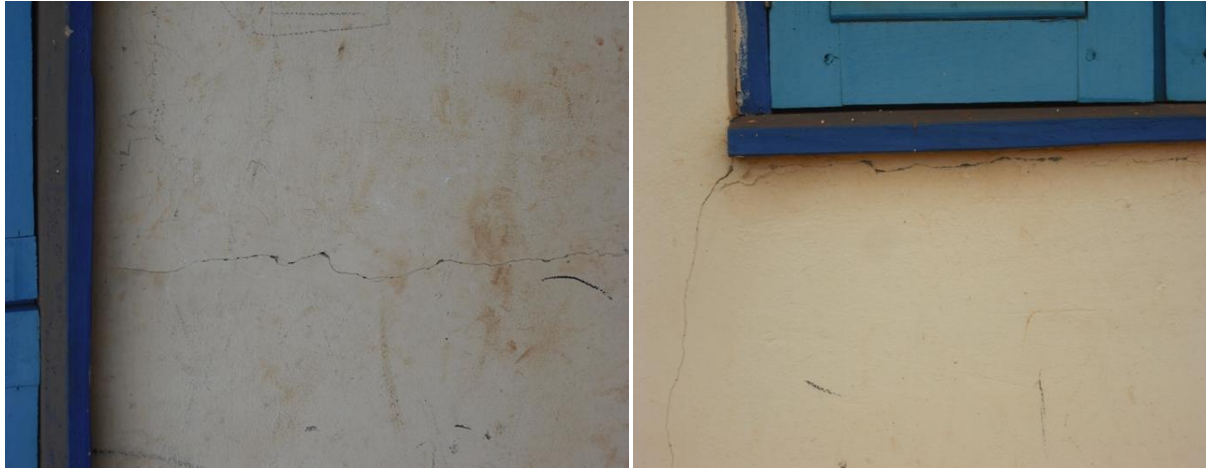
Figure 13. Cracks in some building due to site blasting by Newmont Company. Photo: Researcher, 1 st January, 2010.
