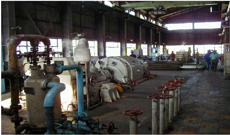
Fig. 8. Boiler and turbine section (photograph by Magne Bråtveit)
