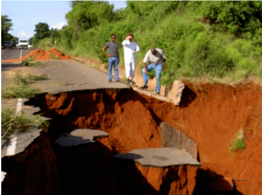
Figure 10: On the way to Guija the rainfall had done something to the road...
