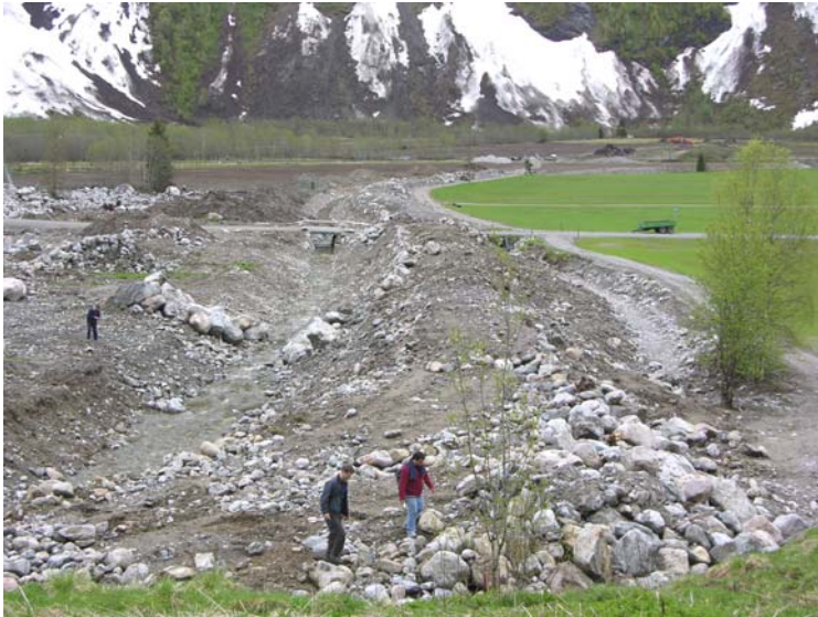
Figure 12.1 Retention and deflecting dam being built between the fan and the farm Øygaard. Photo taken May 2005.
