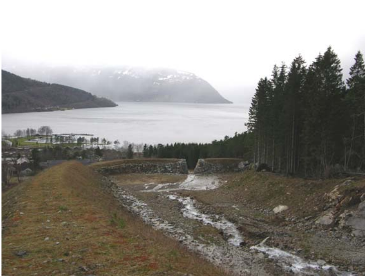
Figure 12.2 Deflecting dam for a debris flow built in Hardanger, Norway. Notice basin and drainage opening.
