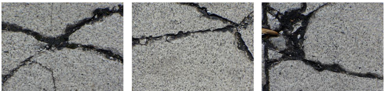
Figure 5: Frames from Test 1 (East London Street)
