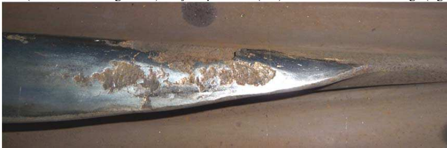
Figure 14. crossing nose showing heavy plastic deformation and distorted nose under the impact of passing wheels (non-compliance of wheel-crossing geometry)
