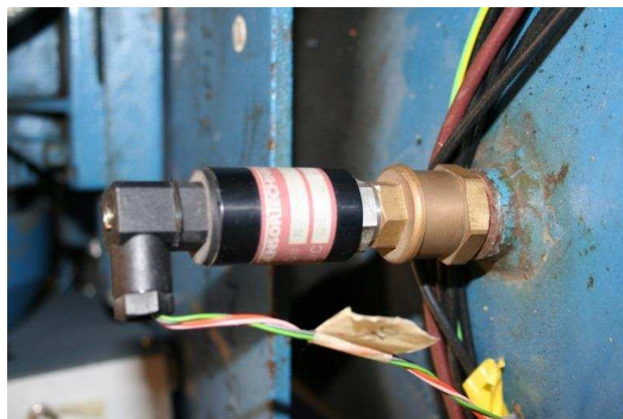
Figure 3.7 Static pressure sensor on air storage tank
