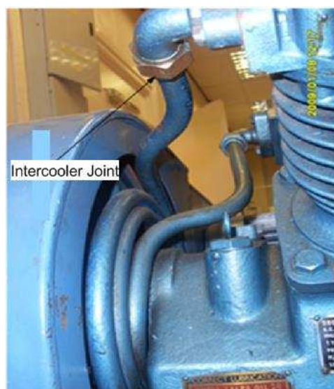
Figure 3.3 Leak in the intercooler
