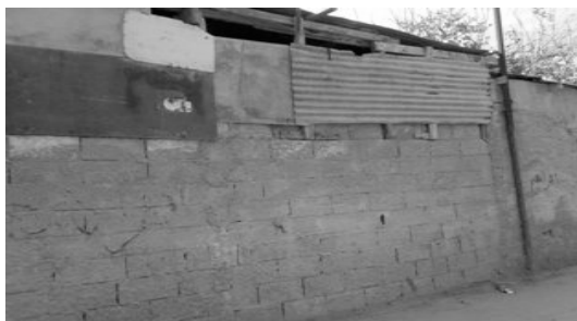
Figure 2 Poor structural quality of houses
