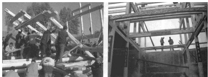
Figure 33: Erecting the timber framework and sticking couplings on the beams and columns (Bin, 2011, p.132)
