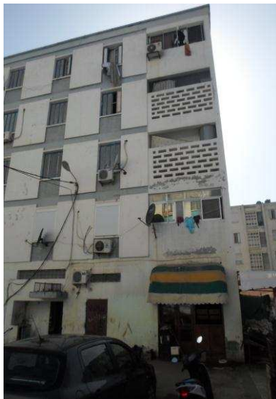
Figure 3: Example of ‘closed’ balconies
