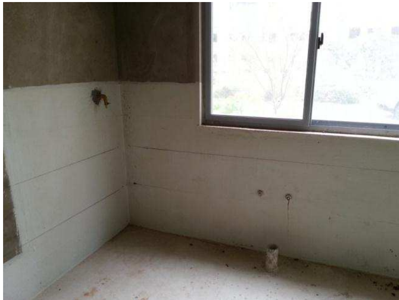
Figure 7. A room in a basic apartment with no systems, appliances or finishes.
