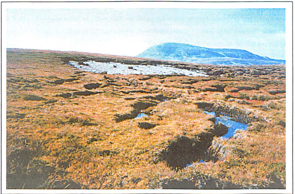
Plate 3.3 Failure scar and subsided cracked bog of bog flow E2 which occurred in August 1992. Cuilcagh Mountain summit ridge to the upper right. (Photo: K.J.K., October 1997).
