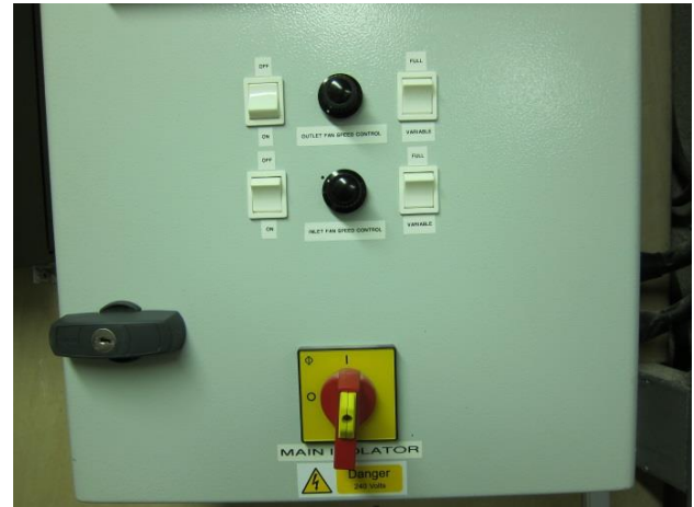
Fig 7: Fan control panel
