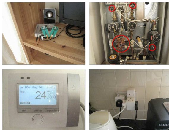
Fig. 7. Examples of home network components deployed in the prototype installation. Starting clockwise from the top left corner, they depict a UWB platform measuring occupancy, Xbees sensor monitoring the boiler operation, a Zigbee HA plug module and a Zigbee HA Thermostat.
