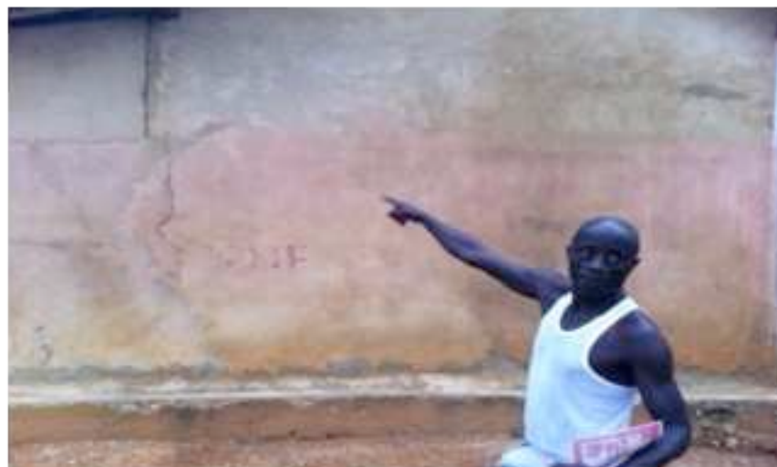
5.7: A Dumasi Community resident pointing out the damaging cracks to one of many houses as a result of the frequent dynamite blasting by the mining company. No compensation or cost of repair has been paid. Source: Author's own (picture used with permission).
