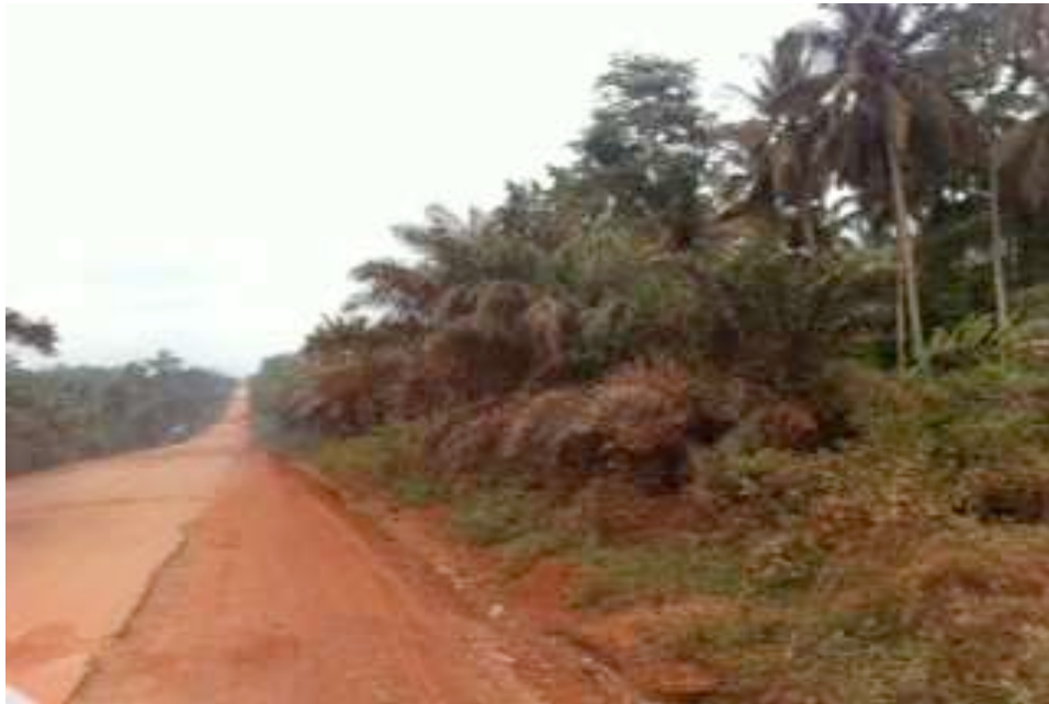
Main road leading to the Dumasi very poorly constructed (half surface tar eaten away) and dusty. Note the Palm fronds and vegetation looking very brown from settled red dusty.
