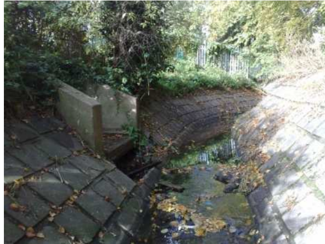
Figure 4.22 View of Mayes Brook at Stretch 1 [MB_001WC] at the time of survey, showing full reinforcement of banks and bed during low or dry weather flow conditions
