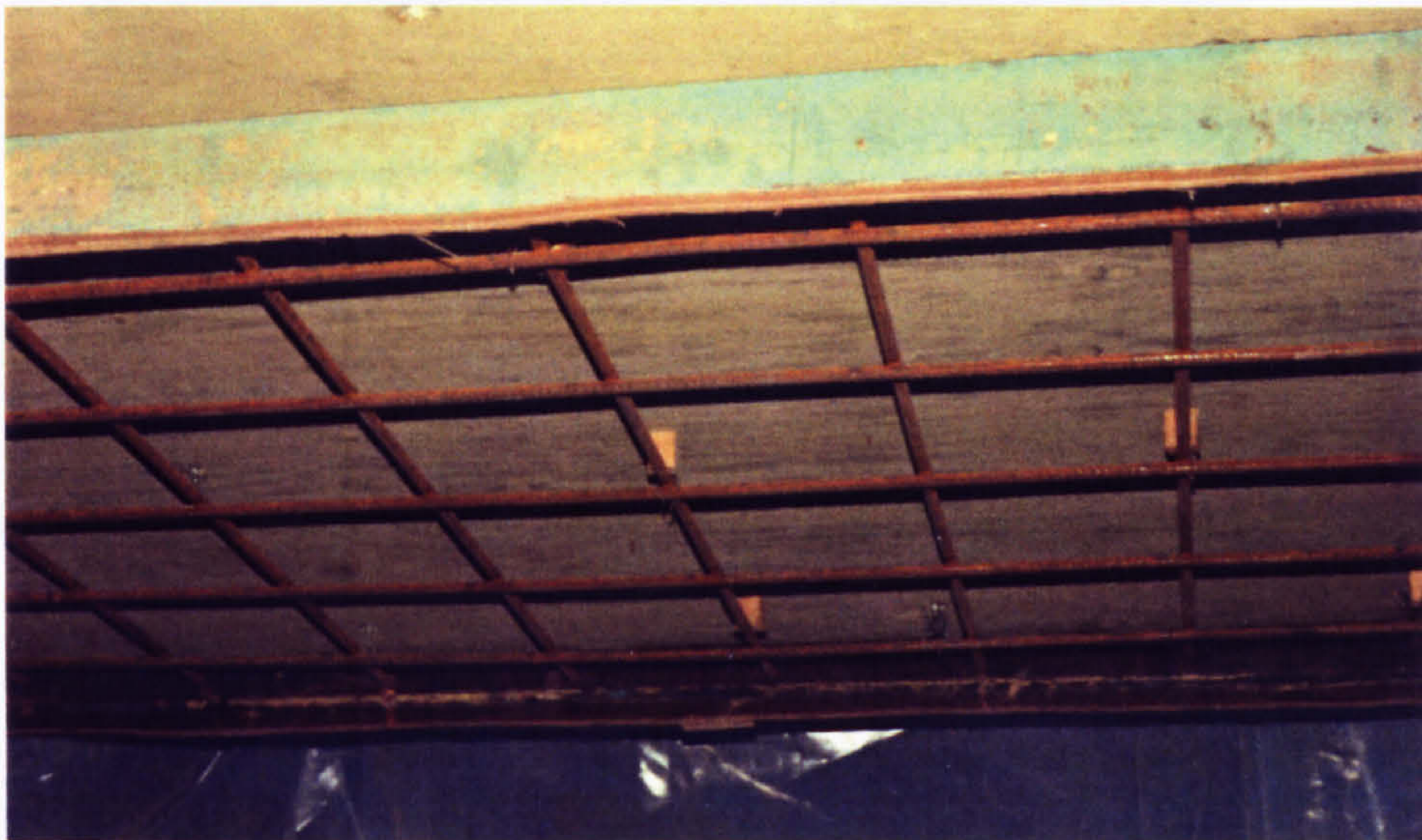
Figure 3.2a - Base slab soffit, formwork finished (the contractor decided to fix the mesh reinforcement before spraying the concrete for this slab).
