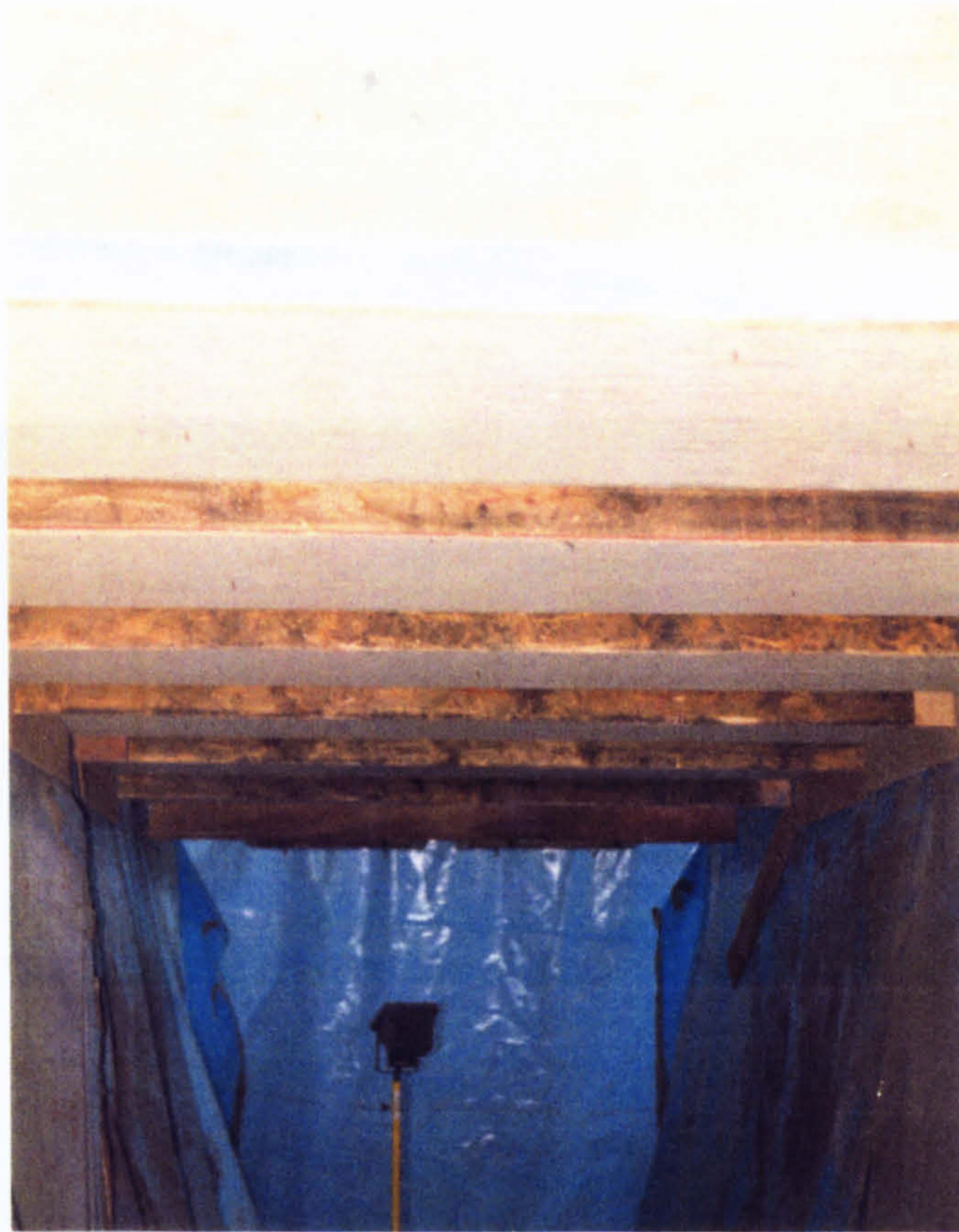
Figure 3.1b - The precast R-C base slabs positioned on scaffolding at two metre height (looking from below soffit level, inside the plastic sheeting).
