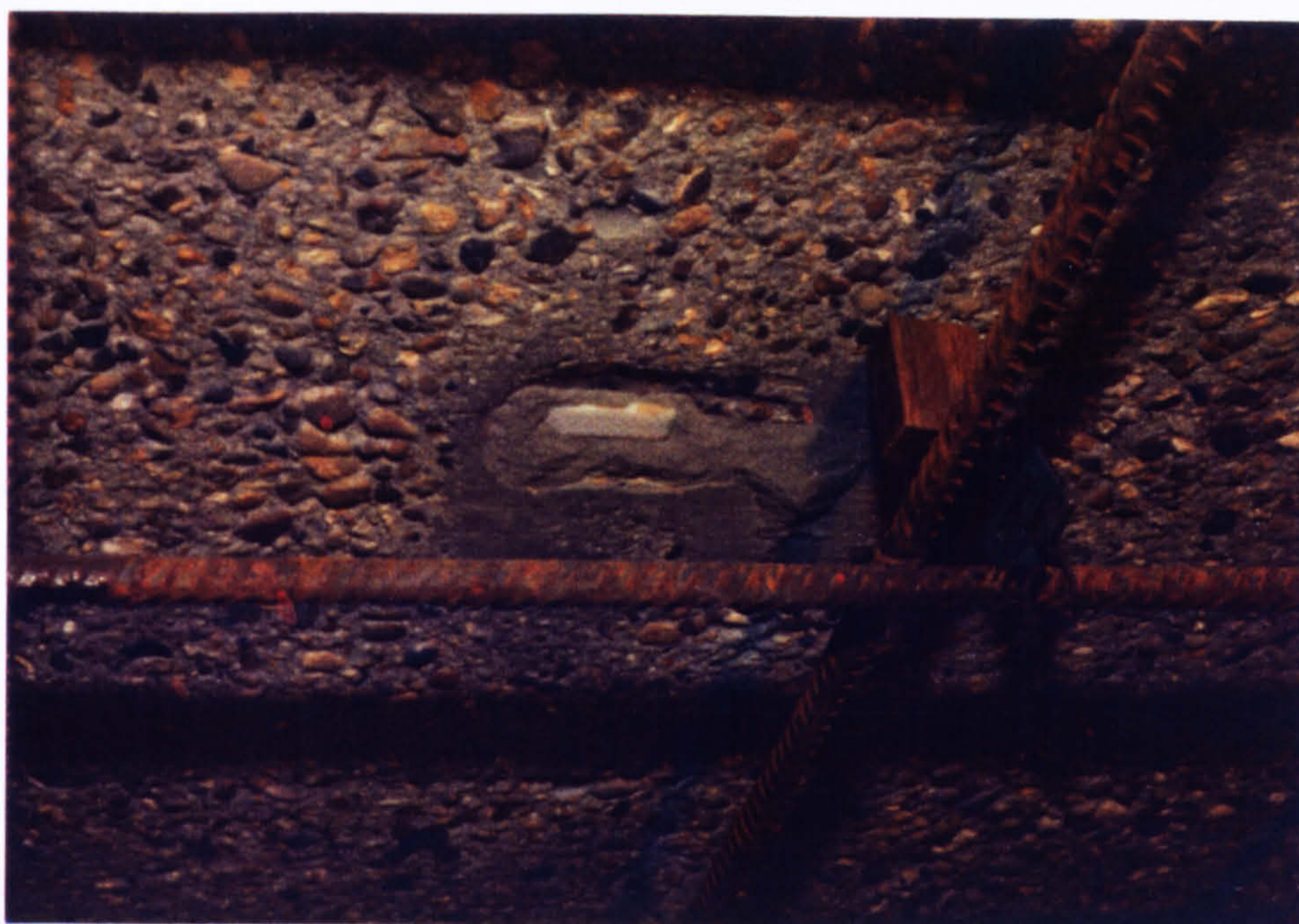
Figure 9.7 - A prepared strain gauge attachment, just before the concrete spraying process (looking from below soffit).
