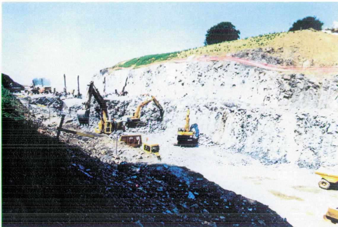
Fig. 7.2 A view of the new rock cutting known as the A5 Glyn Bends Improvement site
