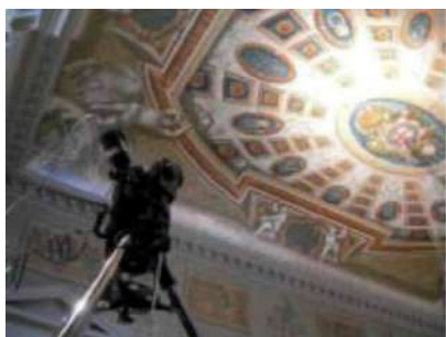
Figure 3. Qualitative remote imaging to inspect the ceiling of the Queen's staircase at Hampton Court Palace using PRISMS.
