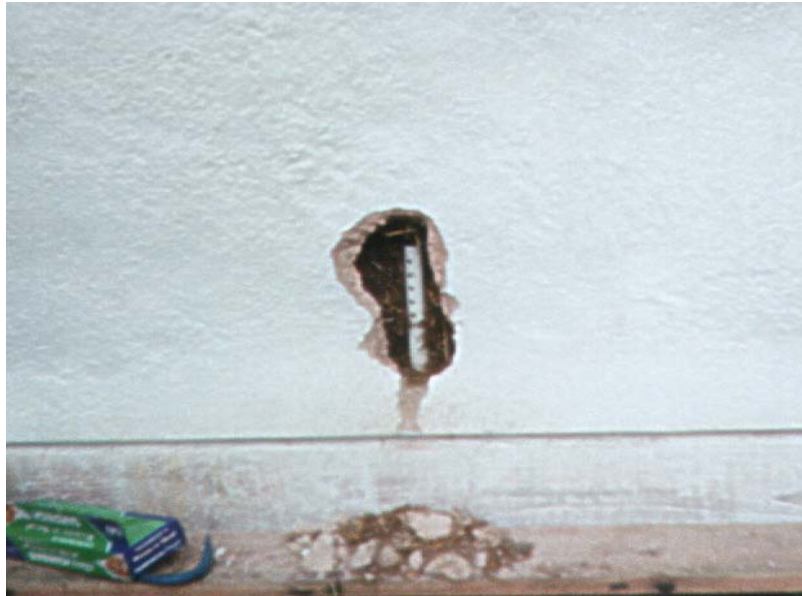
Figure 10, Chipped off render, exposing the probe.
