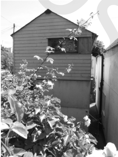
Figure 2. Building one, with a thermal probe inserted in the foundation blocks 120mm below the DPC, supported on a boom stand.
