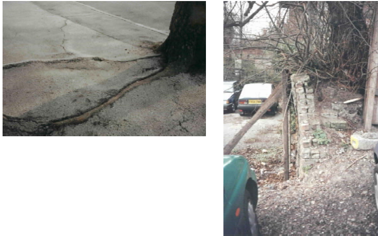
a). Damage to pavements and retaining walls due to tree roots at Nottingham Trent University car park.
