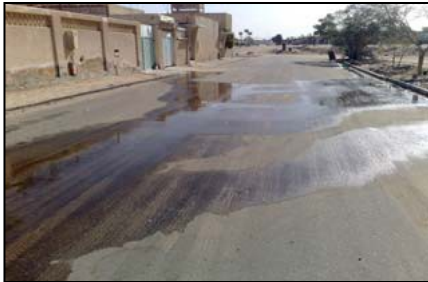
Figure 9: Evidence of urban water waste in Alwihat, 2009 (photo by the author).
