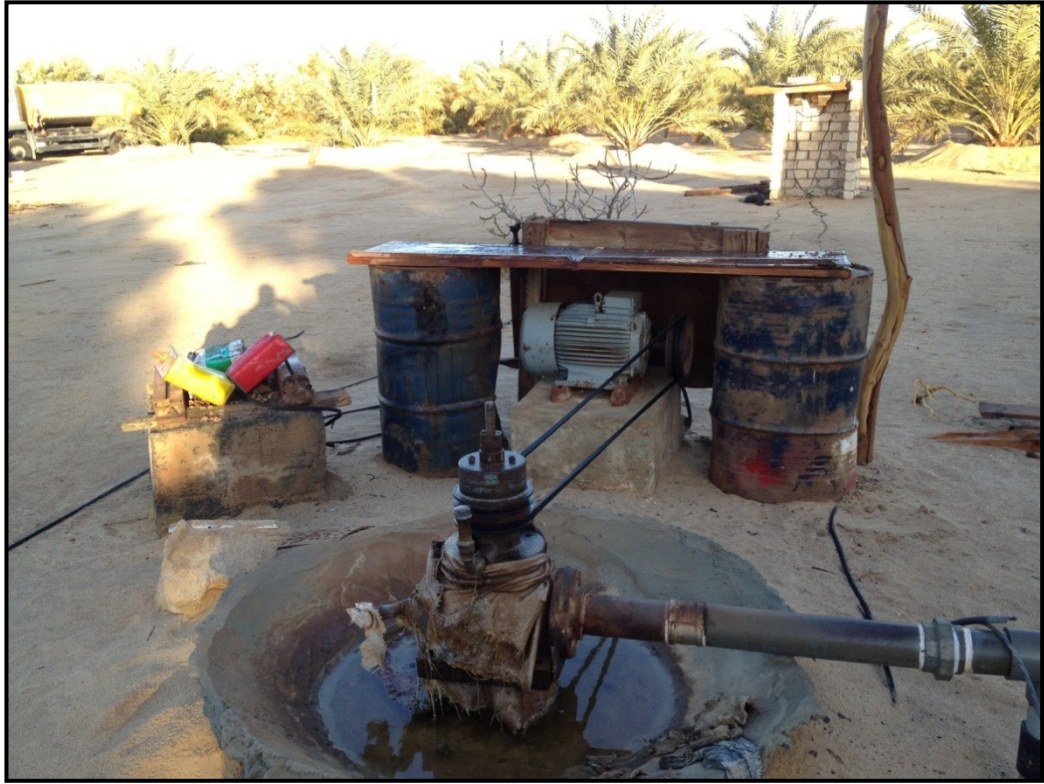
Figure 24: The commonly-used drilling water wells in Alwihat area (photo by the author, 2010).
