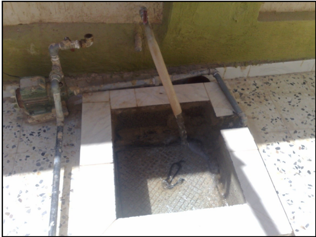
Figure 19: Underground water tank in Alwihat area used to collect drinking water which comes from a municipal water pipe line network (photo by the author, 2010).
