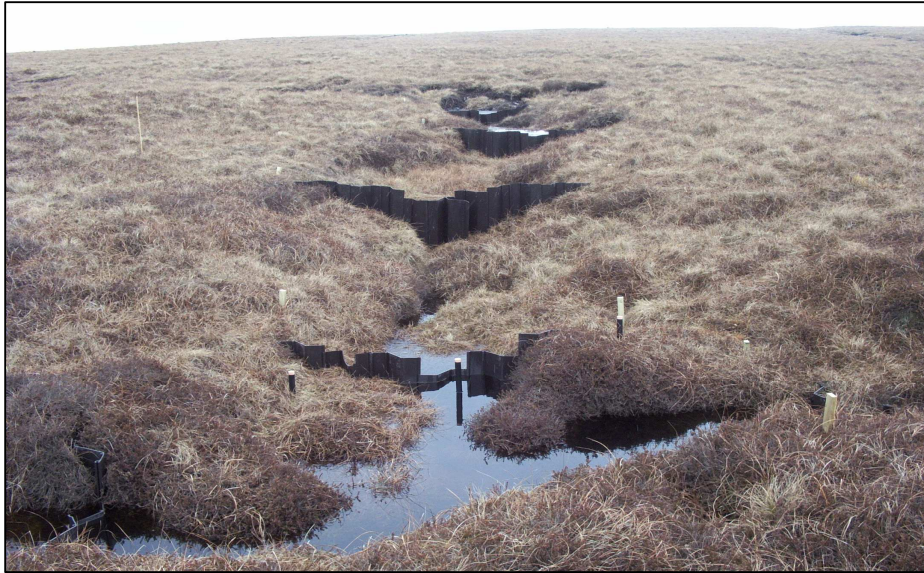
Figure 4.3: Gully blocking with plastic piling at Within Clough, south Pennines
