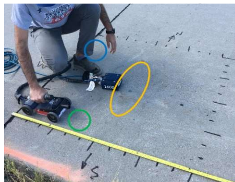
Figure 2.21 Field Experiment 1 - Scanning Grid with Suspected/Detected Voids
