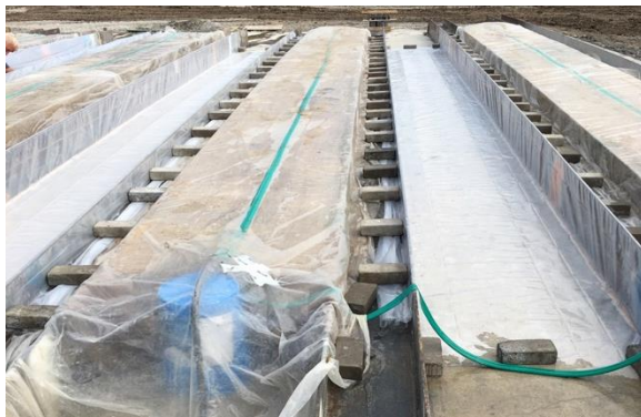
(a) Simple steel forms to cast planks (photo taken at the Midwest Underground Casting Facility in Nebraska)
