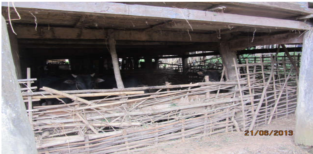
"Cattle house" under the floor of Pole house of Thai people Group 2: Phong Lai Commune, Thuan Chau District
