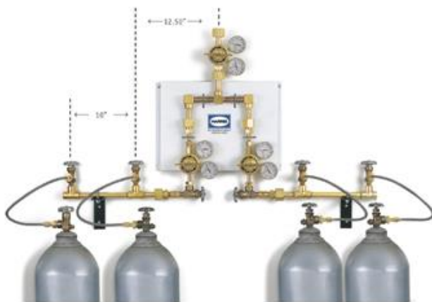
Figure 6: Typical gas supply manifold (Midwest, 2015)
