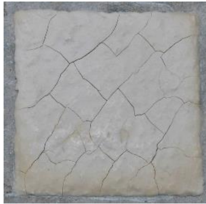
371 372 Figure 10: Cracked patch printed onto dry concrete substrate
