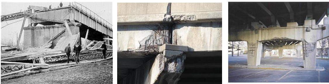
Figure 1. a) Bridge Collapse in Ohio due to corrosion, Public Domain; b) A bridge in Monroeville, Pennsylvania, shows signs of embedded steel rebar corrosion, photo of Anil Patnaik ( http://corrdefense.nace.org ); c) Bridge piers show sign of corrosion [34]
