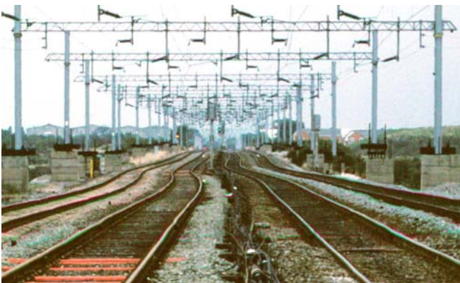
Figure 3. Lateral and vertical movements of the Crewe to Manchester railway line over an area of active salt dissolution and subsidence. Note the pylon bases with vertical adjustment and the lateral movement of the railway line. Photo A.H.Cooper © NERC.
