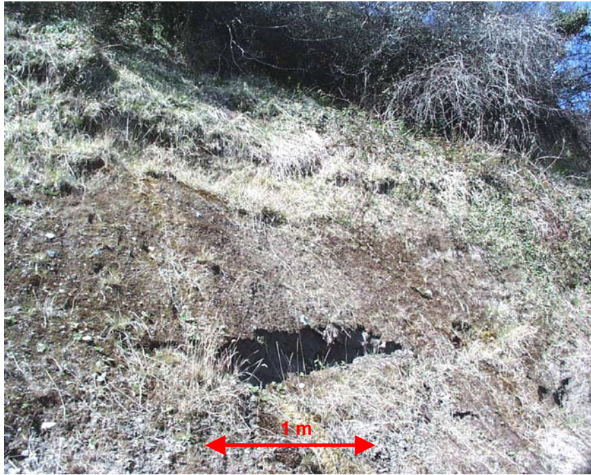
Figure 7. A shallow failure within the exposure of poorly laminated gravelly silt 10 m NW of the exposure in Figure 6., (looking NNE at approximate grid reference [223774, 328156, z34].
