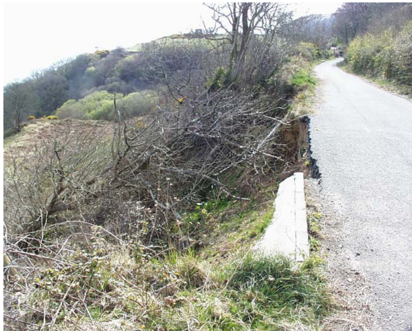
Figure 20. Loss of kerbing and road surface due to undermining southwest of Sarn y Plas.
